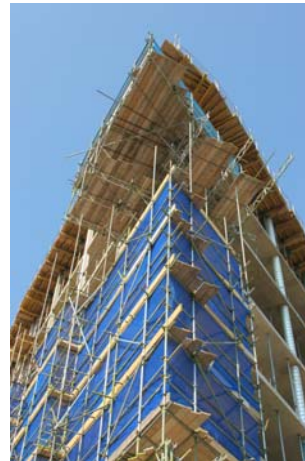
New building for the Faculty of Arts University of Plymouth, Plymouth, Devon
